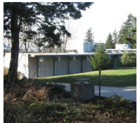
MULTIPLE ROOF FAILINGS
