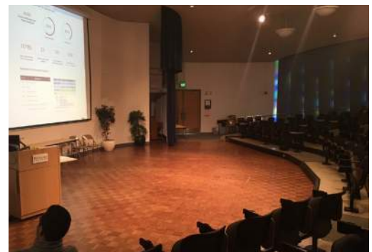
EXISTING WOOD FLOORING TO BE REPAIRED/REPLACED
