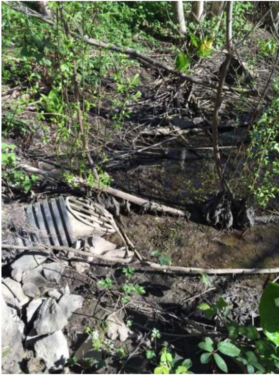
1. Outlet pipe from second cell
