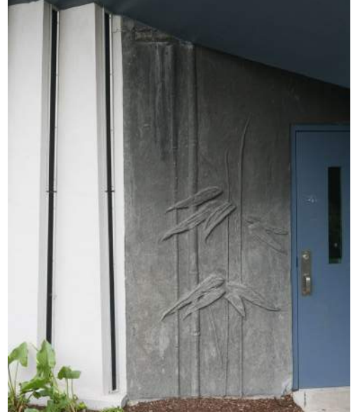
Right: Detail of panels, Building 7. All contemporary images courtesy Artifacts Consulting, Inc., 2016, unless otherwise noted.
